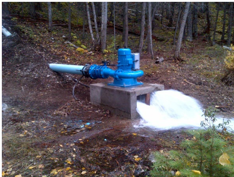
Figure 7-4: Micro hydropower facility (Source: Suneco Green Energy [8])
